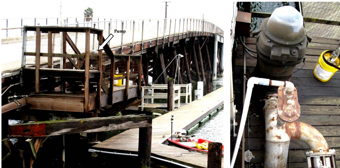
Abandoned Pump Intended for Fire Protection of Bethel Island's Business District
