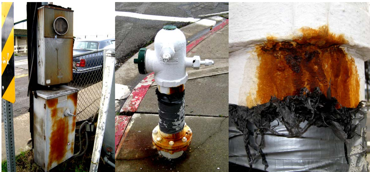
Abandoned switch meter box for pump, and an unused corroded fire hydrant in the business district
