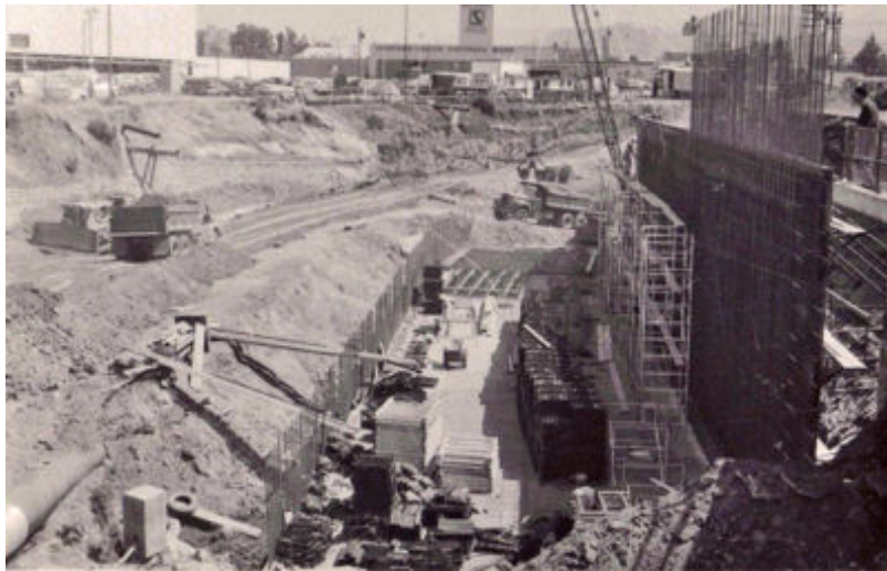
Construction of the culvert under Broadway Plaza in the early 1960s (Courtesy of the Walnut Creek Historical Society)
